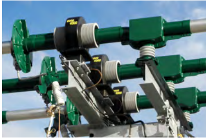
AltaLink Current Transformers and Bus
