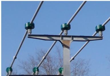
Middle Tennessee utilizes Greenjacket expansion joint covers to prevent animal and bird outages.
