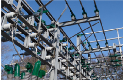
Brentwood Substation distribution bay breakers and angle bus supports protected with Greenjacket.
